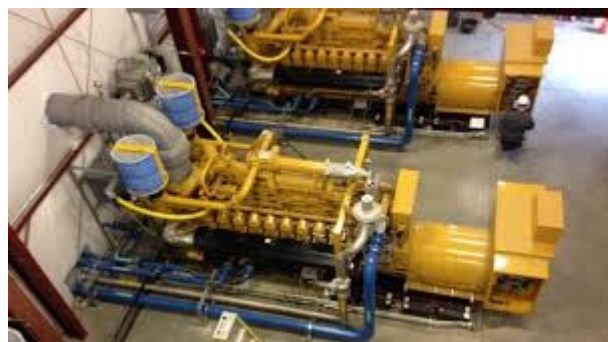
Figure 1: A Caterpillar 3520C stationary generator
